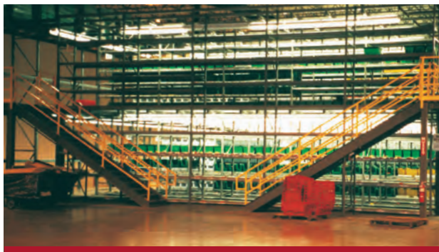
Multi-level Wide Span Pick Module
